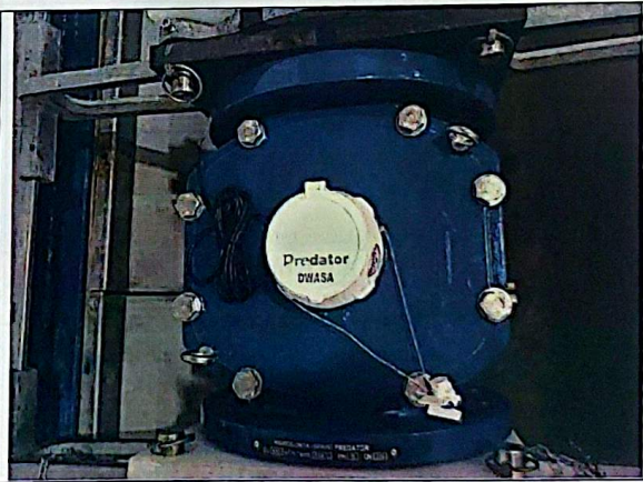
Water meter with seals
