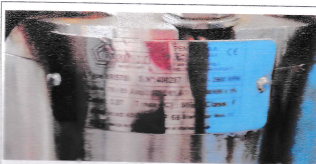
No. 27 – Nameplate motor S/N400287
