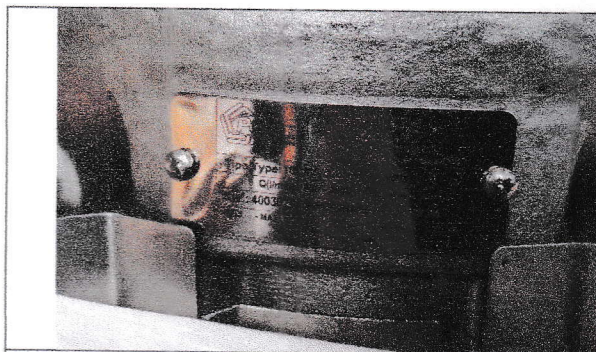
No. 15 – Nameplate pump S/N400302
