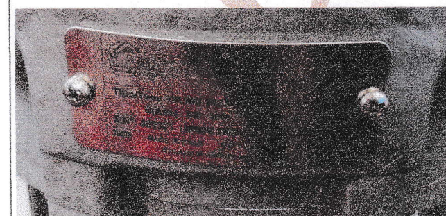
No. 13 - Nameplate pump S/N400301
